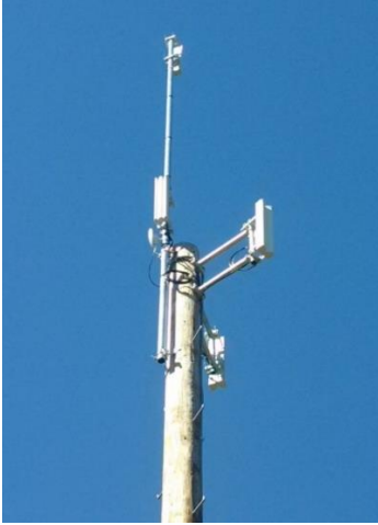
Figure 2: Antennas on top of 50' pole in Royalston.
