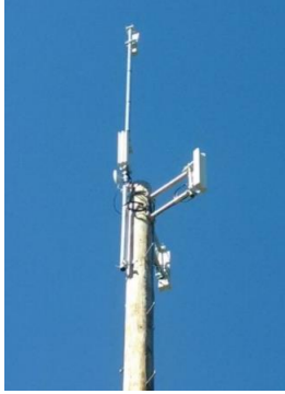
Figure 1: Antennas on top of 50' pole in Royalston.
